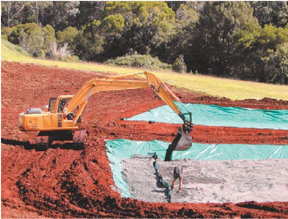
As part of a research project, two reed beds were constructed to clean runoff water at Bau Farm Wholesale Nursery on the New South Wales north coast. Each was 150 cubic metres, sealed with heavy-duty plastic and filled with five millimetres of blue gravel.
