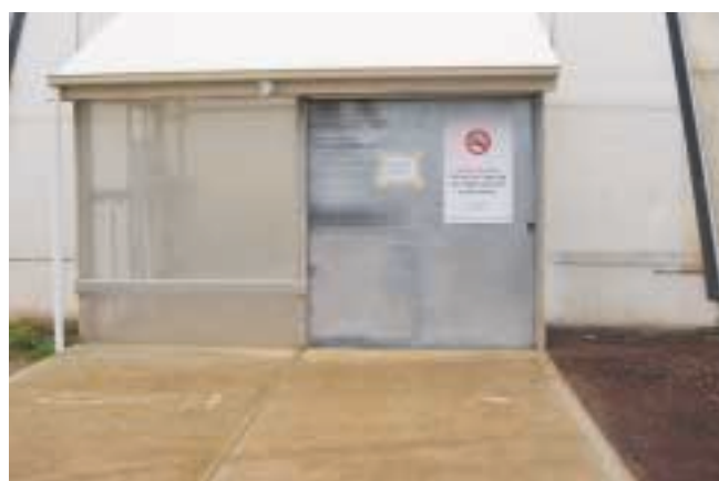
A double entry door with fine mesh and an outward directed fan that operates every time the door is opened can significantly reduce pest incursion. Virginia Horticultural Research Centre, SA.
