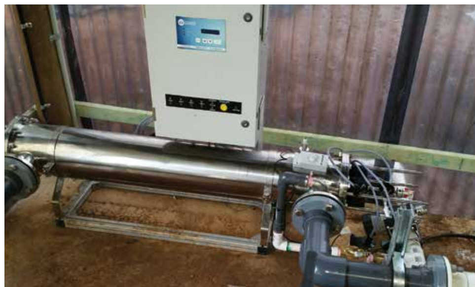
New UV generator being installed
