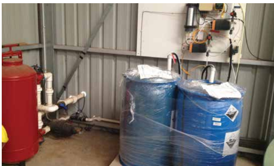
Chlorine dioxide generator
