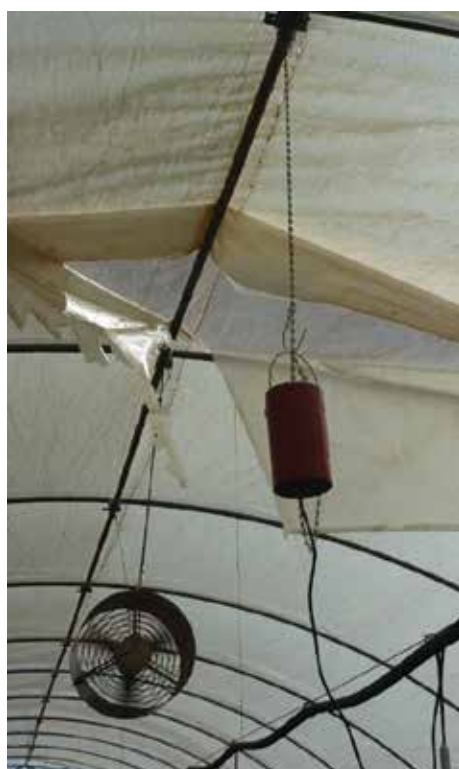
A sulphur diffuser hung at an incorrect height and aided with fan dispersal but destroying the plastic covering above as it is too close.
