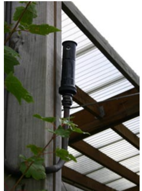
Essendon Garden Centre uses this efficient gear driven sprinkler as part of its automatic sprinkler system.
